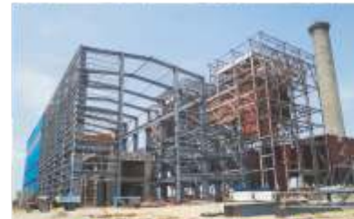
BHARAT TURBINE ROOM, INDIA
